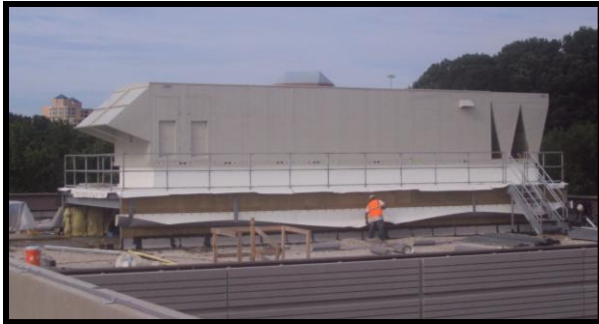
Figure 5: Roof Top Air Handling Units
